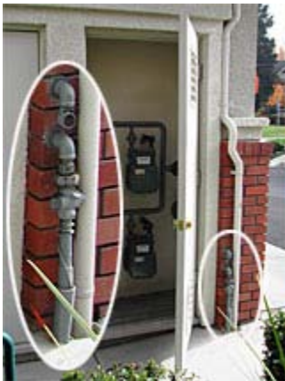
Cabinet Meter Outside
