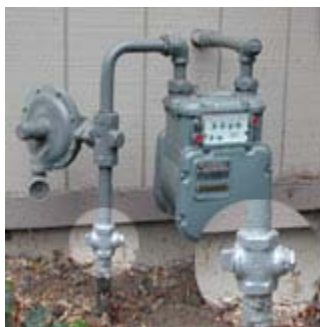
Gas Shutoff Valve
